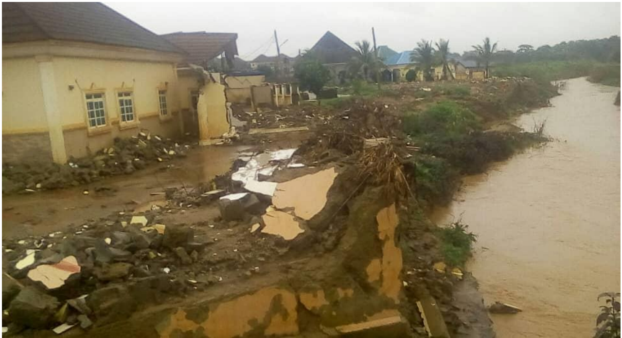
Fig. 1.5: Property erected along river courses that were destroyed by flood in 2019.
